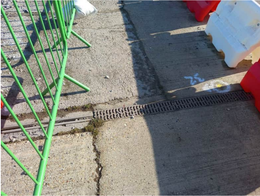
Photo 31: ACO drains at HZI construction site.
